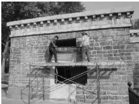
Work underway on the gatehouse at the Bronx end of the High Bridge. (Courtesy of the NYC Dept. of Parks & Recreation)
