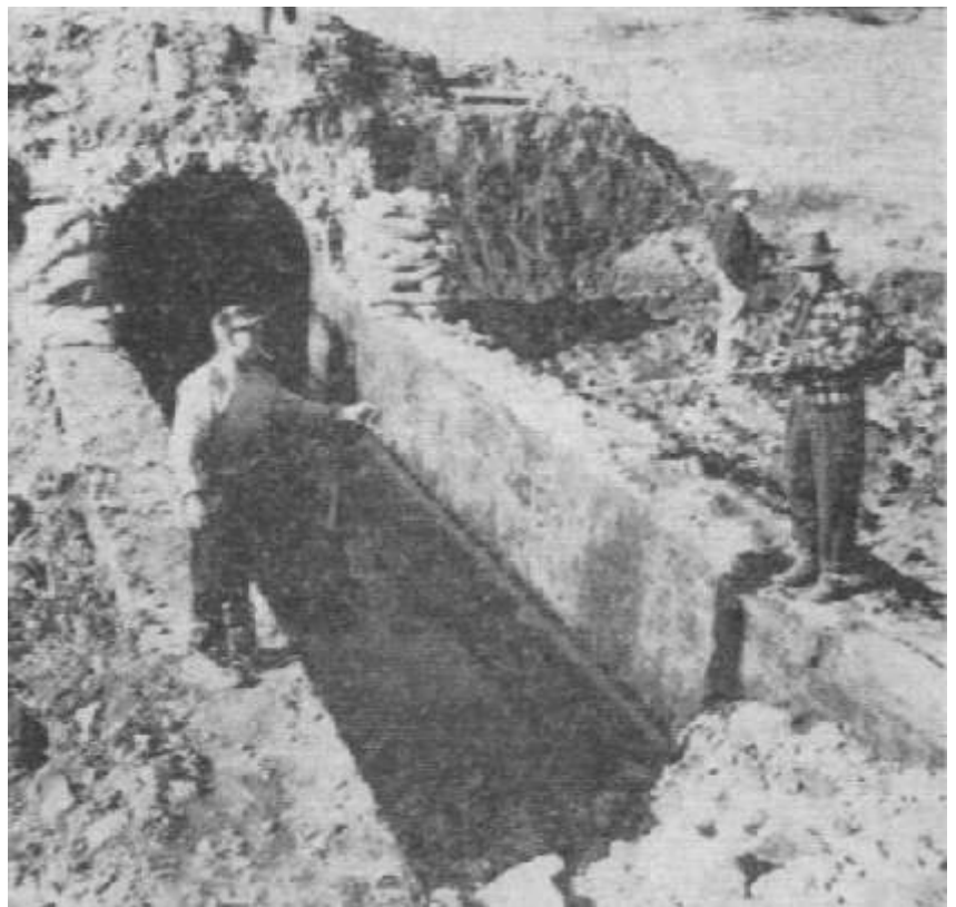
"Croton Aqueduct had to be reinforced with steel pipe during construction of the New York State Thruway. Here workmen measure the gap across the aqueduct to fit the pipe. Use of the pipe will prevent collapse of the aqueduct when traffic starts using Thruway. - Photo by Dan Berry." 1955. (News clipping courtesy of the Historical Society of Sleepy Hollow and Tarrytown)
